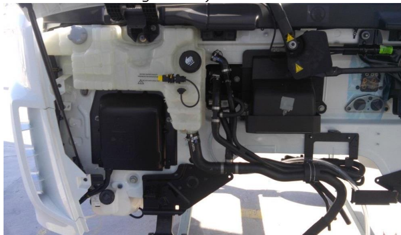
Figure 26 Electrical Junction Box Location
